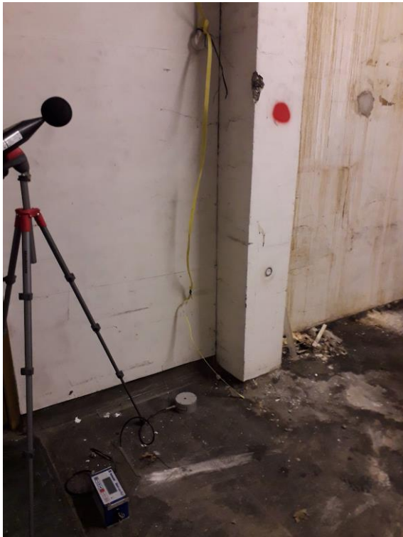
A3.2: Test No. 2 – Boring Holes to Coring Column, Lift Shaft, Ground Floor.
