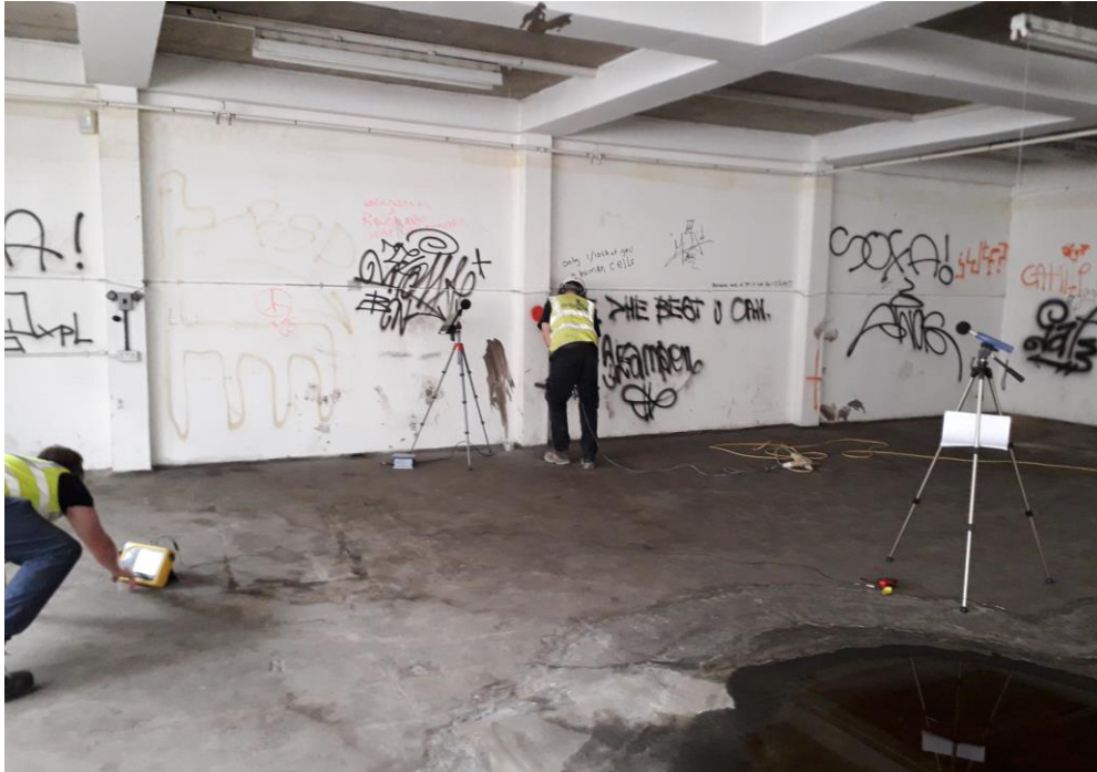
A3.7: Test No. 7 – Boring Holes to Coring Column, Front Room, First Floor.
